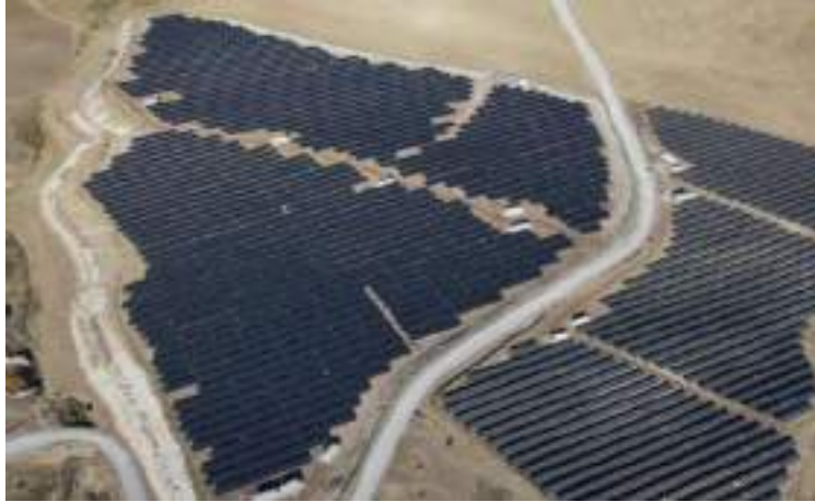
Fig. 1 Solar power plant
