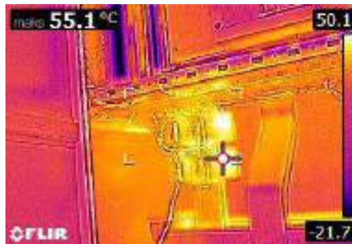
Fig 5. Image of current transformers overheating and their bodies cracking
