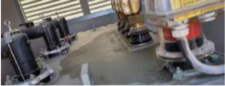
Fig. 6 Real image of bushings in transformers
