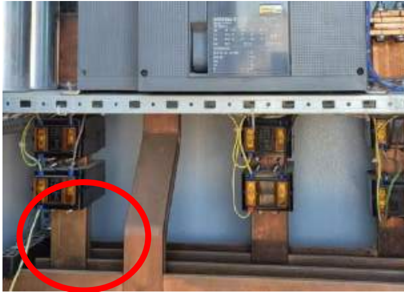
Fig. 8 Current transformer image
